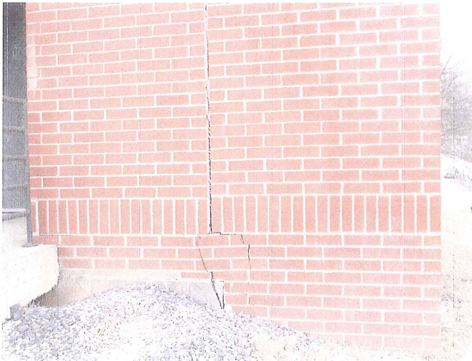
PHOTO 20 - Settlement of Wall Left of Corner
