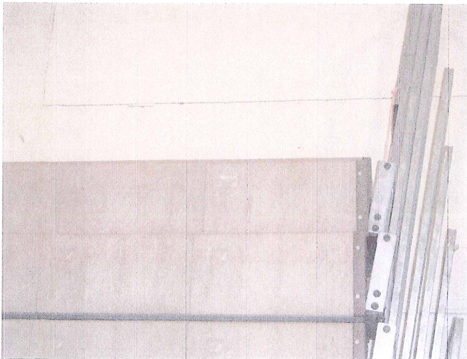
PHOTO 22 - Horizontal Crack Above Bleachers (Close Up of Photo 21)
