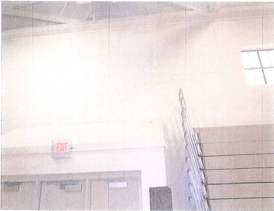
PHOTO 21 - Horizontal and Diagonal Cracking Above Bleachers
