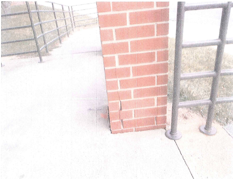
PHOTO 6 - Crack In The Left Brick Column at Stairs Shown In Photo 5
