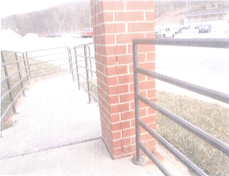
PHOTO 7 - Crack In Right Brick Column at Stairs Shown In Photo 5
