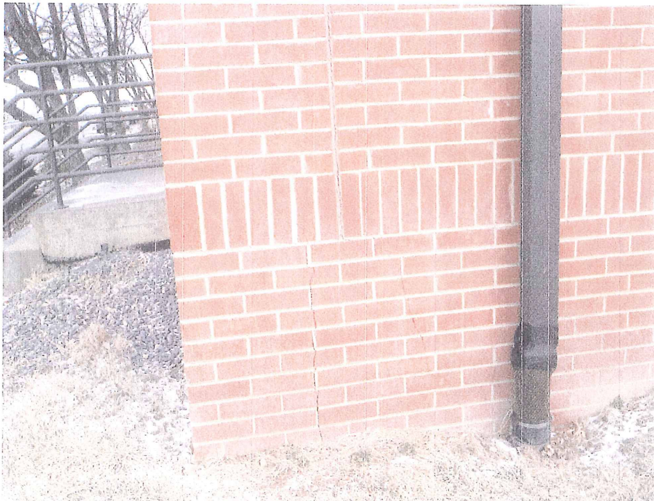
PHOTO 18 - Downspout is Likely Cause of Settlement At Corner
