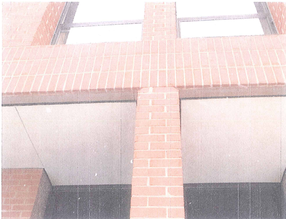
PHOTO 4 - Typical Damage Due to Thermal Expansion / Contraction of Beam
