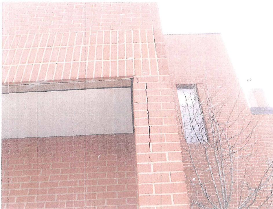
PHOTO 2 - Far Right Brick Column At Front Of Structure Showing Movement Due to Expansion
