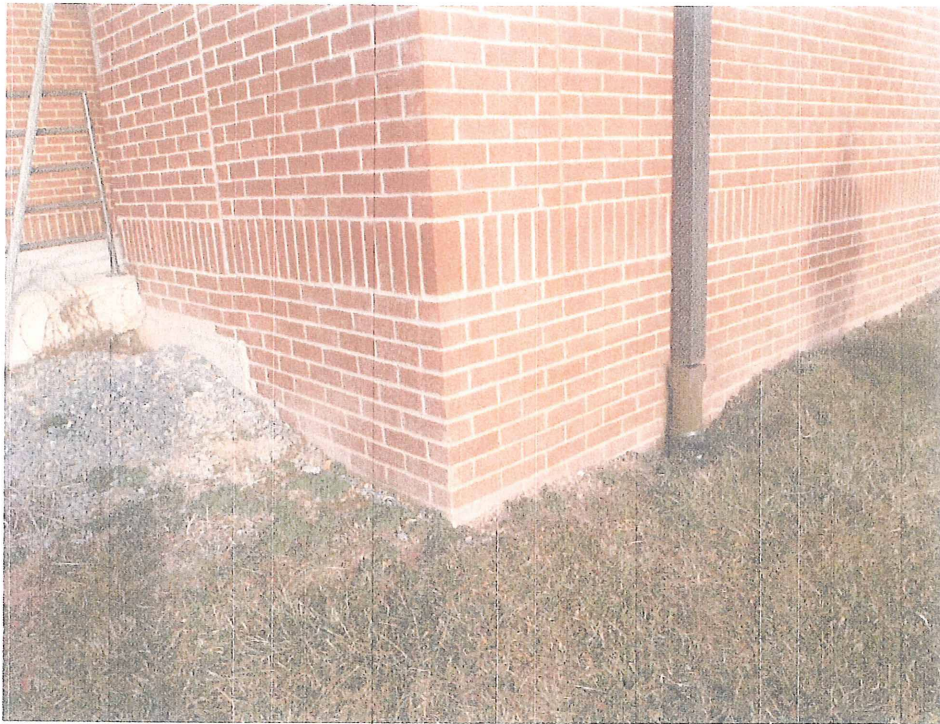
PHOTO 17 - Gymnasium Corner Showing Differential Settlement
