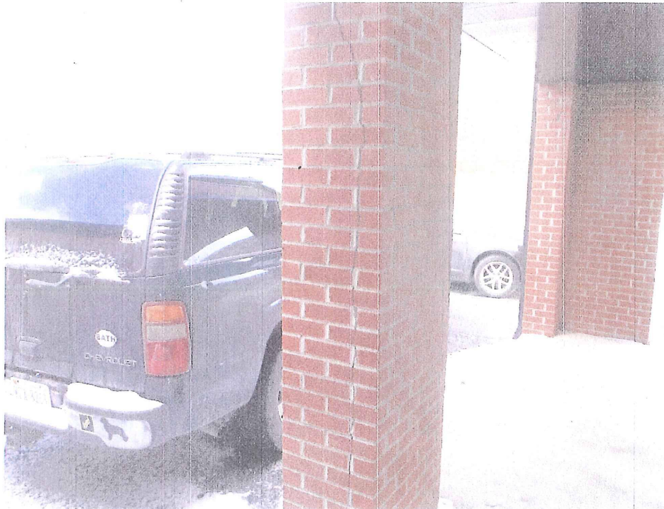
PHOTO 16 - Vertical Crack In Brick Column
